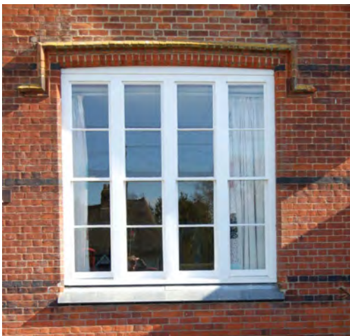
Picture 1.8 Quality window joinery and brickwork evident on the Old School in Crow Street
