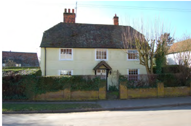
Picture 1.14 Decorative pargetting applied to the Manse. It is highly important that this is retained
